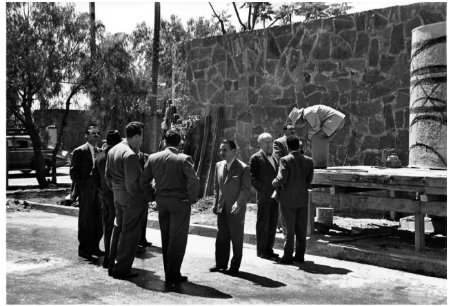
05 Mario Pani, Centro Urbano Presidente Alemán , Mexico City, Mexico, 1947-1949. José Clemente Orozco on the scaffolding, talking to José Villagrán García and José Luis Cuevas, and Mario Pani looking towards the camera, 6 th September 1949, at the entrance of the complex. © Archive Louise Noelle.
