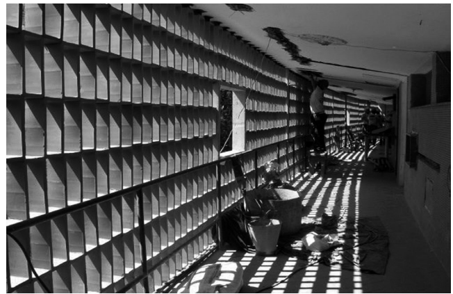
04 Afonso E. Reidy, Carmen Portinho, Pedregulho Housing Complex, Rio de Janeiro, Brazil, 1948-1960. Alfredo Britto, restoration, 2005-2015, Block A, New cobogó panels viewed from the interior. © Alfredo Britto, 2015.
